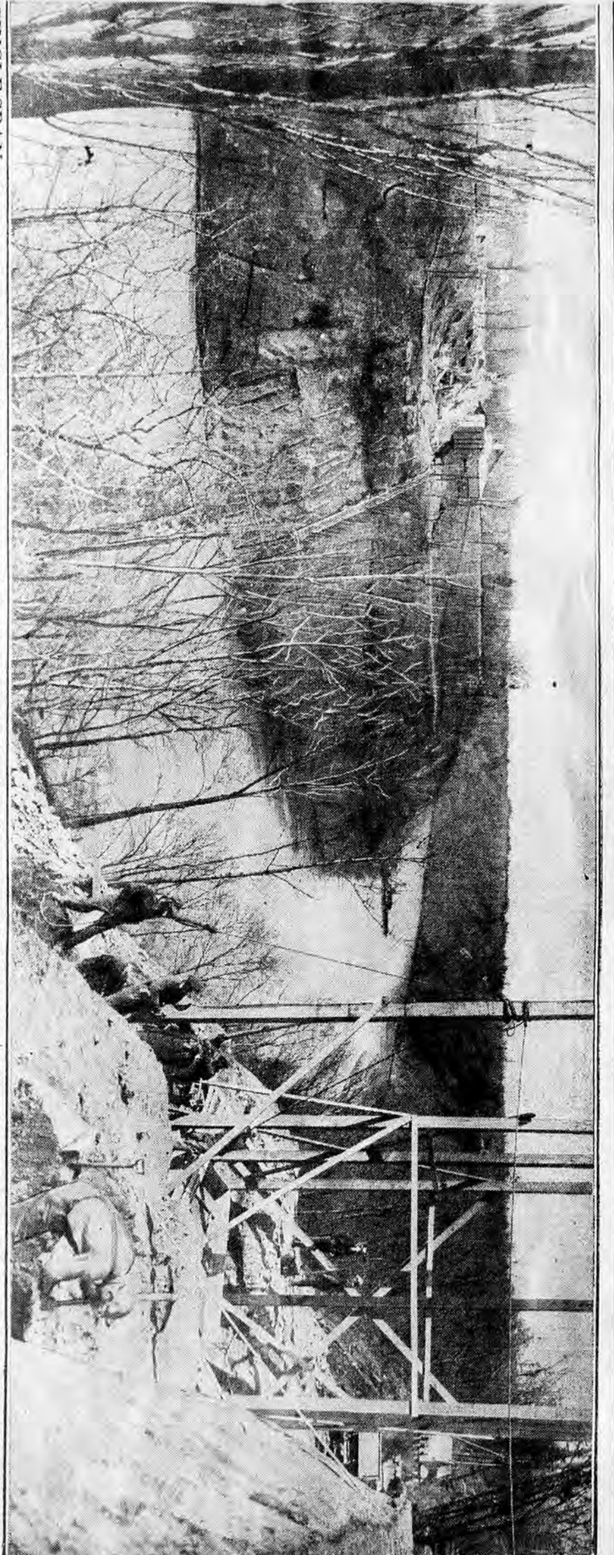
SINGLE SPAN—From the point at the right where workmen are engaged in building foundations for the new Ridge Road bridge over the lower river to the left where the western end will rest the bridge the approaches from east and west. The bridge will be completed some time in the summer of 1931.
